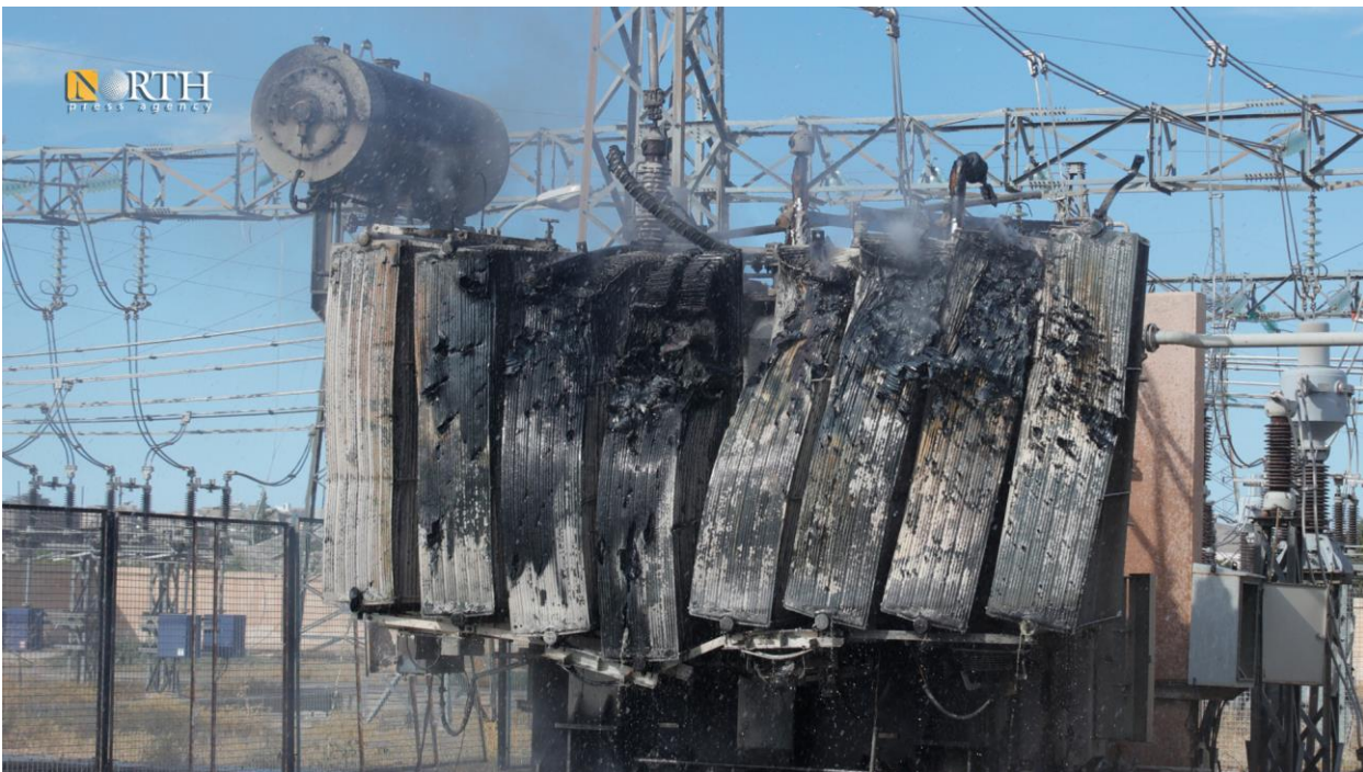
Site 2: The Qamishli power station was completely put out of service after being targeted by drone strikes for three consecutive times 2
