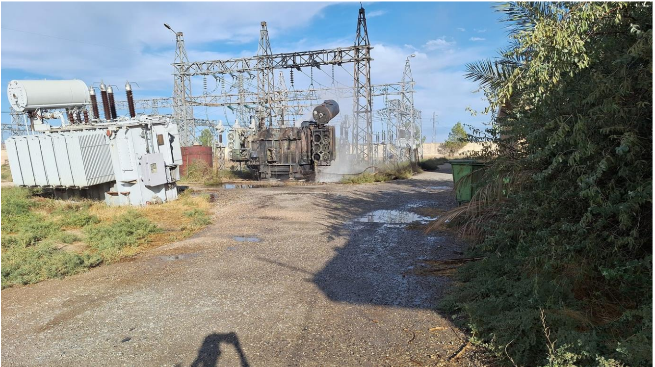
Site 4: The electricity substation in the city of Amuda was put out of service by a Turkish drone strike
